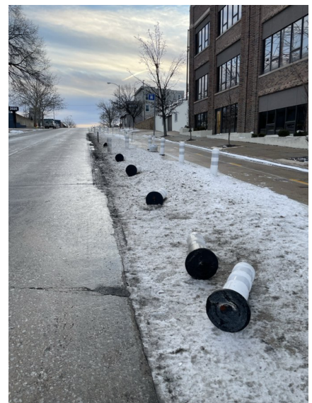
Image 7: Delineator posts became detached from the bikeway due to weather impacting the effectiveness of the epoxy
